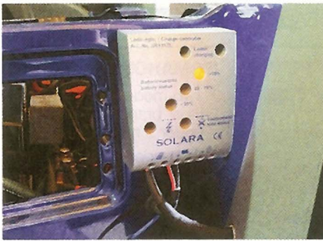
Regulator for the solar panel fitted to side of seat base
