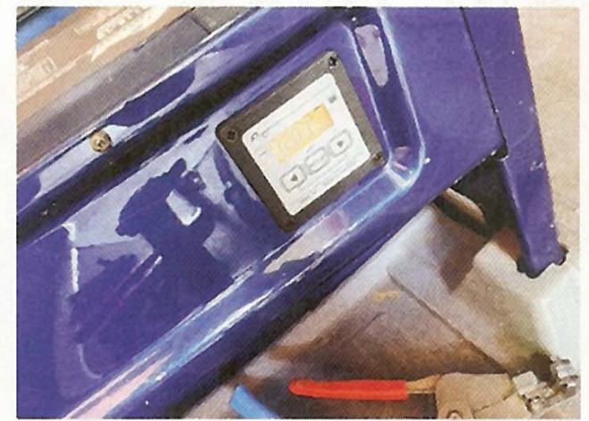
This display allows the battery level to be monitored
